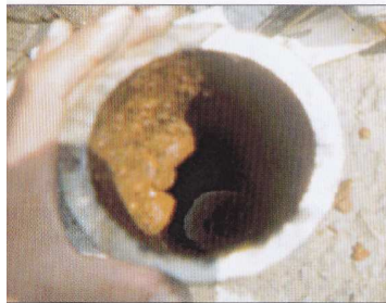
before the installation (October 17, 2002)
